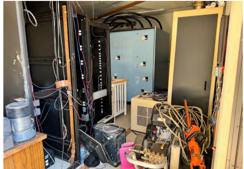
Shed, pad-mounted transformer, and former radio station building
